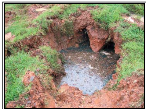
Failed Septic System
