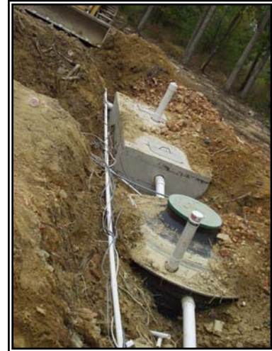
Alternative On-site Sewage Disposal System
