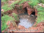
Failed Septic System
