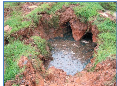
Failed Septic System
