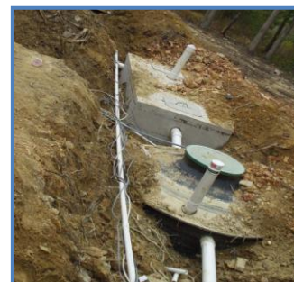
Alternative On-site Sewage Disposal System
