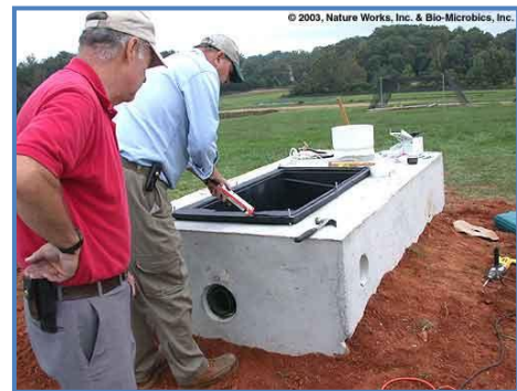
On-site Sewage Disposal System
