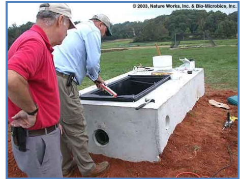
On-site Sewage Disposal System
